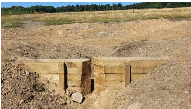
Fig. 4 Whirlow Brook attenuation pond
