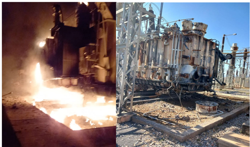
Figure 6. Fire at the Tekeze substation due to drone attack (own photograph in the aftermath of the attack).
