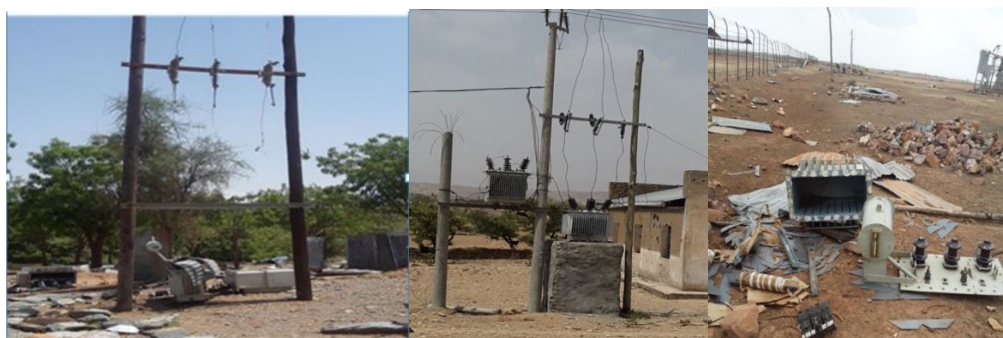
Figure 13. Damaged on distribution systems (authors photo and elaboration).
