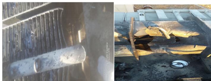
Figure 7. Damages on the Mekelle substation due to drone attack.
