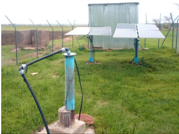
(a) Solar PV panels powering water pump
