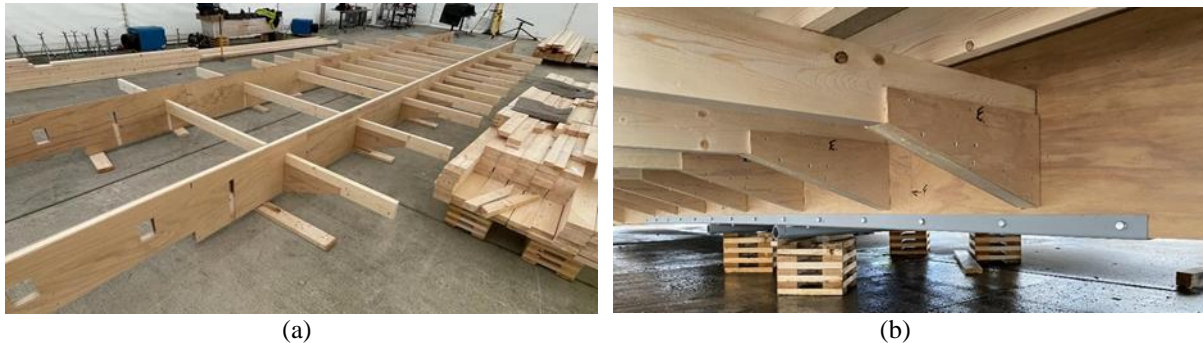
Figure. 11. (a) The assembly process of the wooden chassis, (b) Constraint condition for the wooden chassis.
