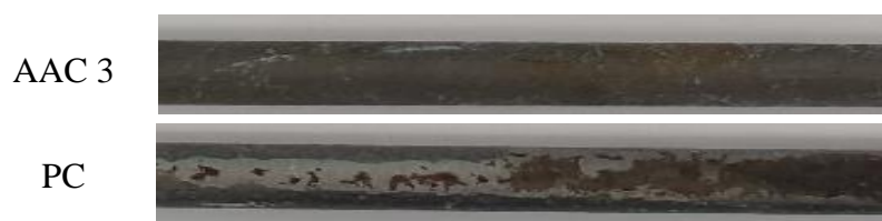
Figure 4: Corrosion of steel reinforcement in AAC 3 and PC concrete after 1750 days exposure
