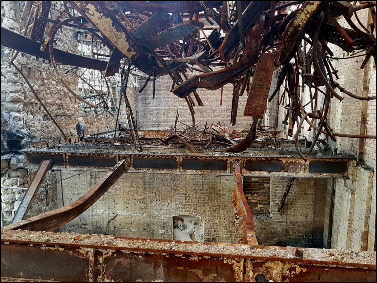
Figure 1. The interior of the Mackintosh Building at Glasgow School of Art following the 2018 fire. Note the distorted steel beams in the foreground; the hanging debris above and the badly damaged stonework on the left. The intense heat of the fire consumed the majority of interior fixings and finishes, leaving the brickwork exposed in most locations.
