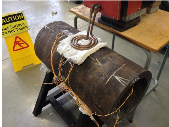
Figure 7 Induction heat treatment of the pipe after completion of the WeldCore® process.
