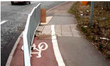
Fig 1. Example of conflict between design standards
