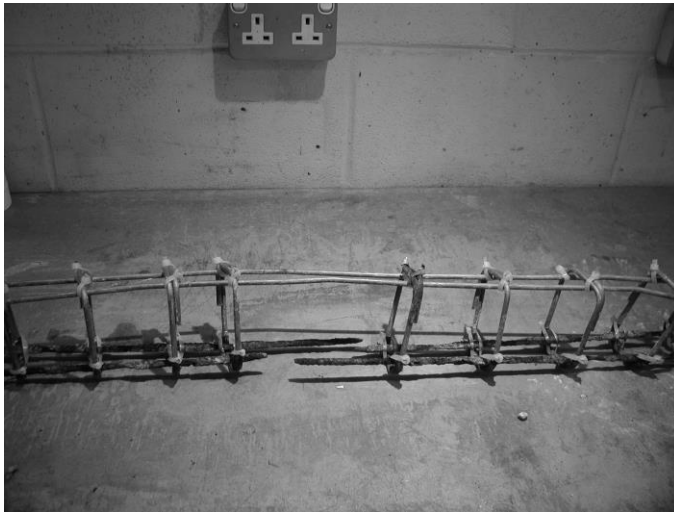
Figure 4. Deteriorated main steel (anode) with uncorroded links and hanger bars (cathode).
