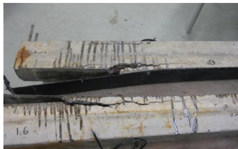
Fig. 10 Debonding of CFRP fabrics after load testing
