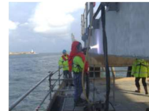
Figure 1 Photograph Showing Application of a Thermal Spray Coating to a Concrete Structure
