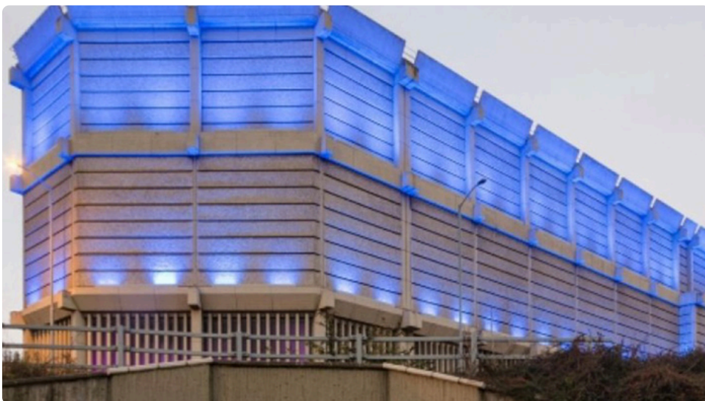
Moore Street substation
