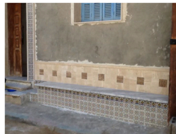
D- The traditional use of built-in bench Rikkaba for male neighbours' gathering, Tripoli, Libya.
