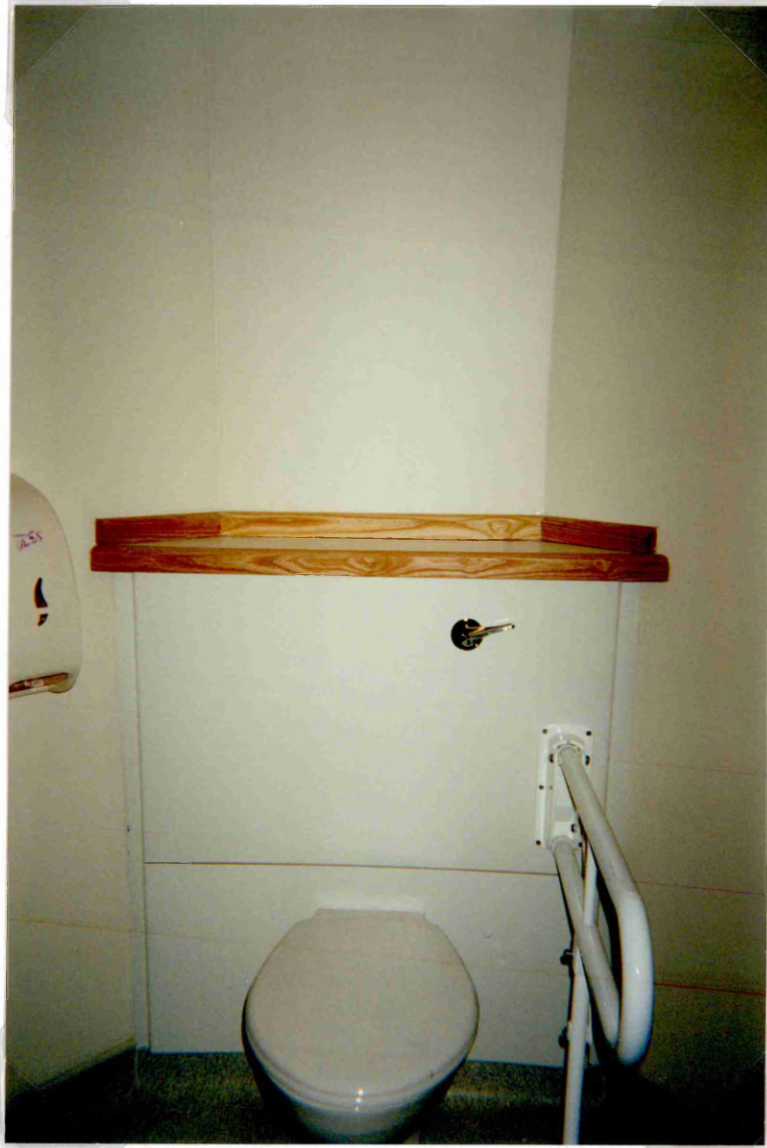
Figure 6.5: WC access panel
